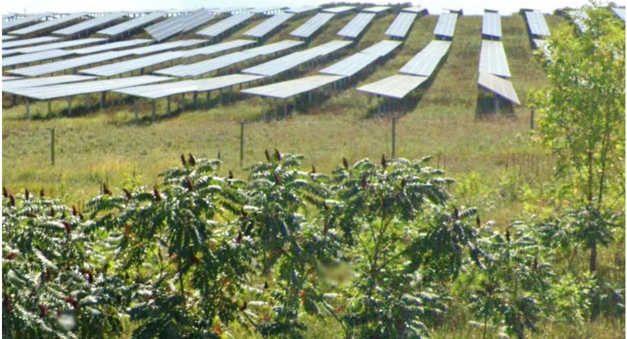
West Waconia Solar – View from HWY – Carver County MN
